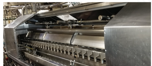
CAN FILLER SERVICE & INSTALLATION
