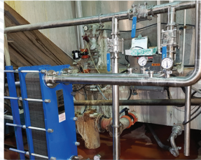
COOLING TUNNEL HEAT EXCHANGER
