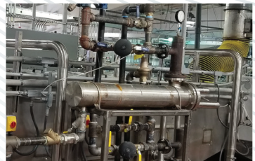
DESIGN MANUFACTURE NEW STEAM EXCHANGER FOR COOLING TUNNEL
