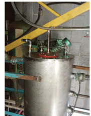
NEW SYSTEM TANK
